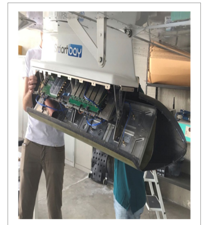
(f) View of fiberglass pod containing the system
